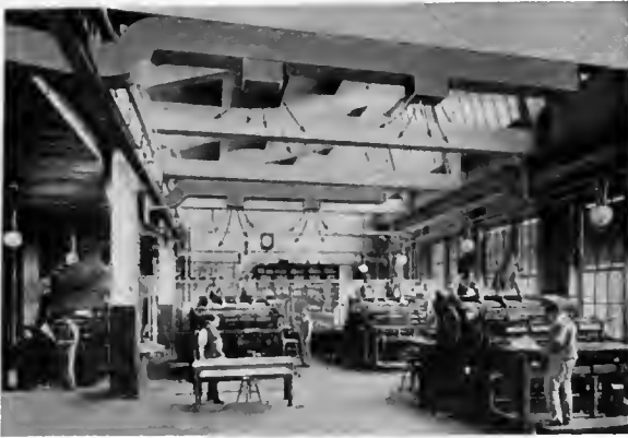
HOT-BLAST SYSTEM INSTALLED IN PRINTING ESTABLISHMENT
